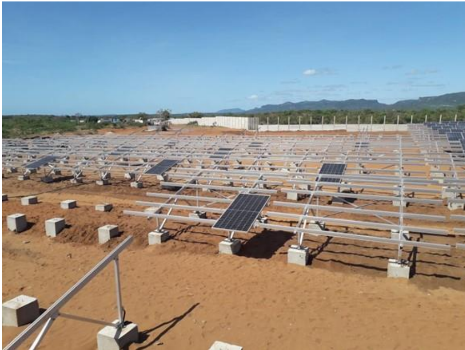
Photo 3 - Solar PV plant with aluminum structures and concrete blocks.
