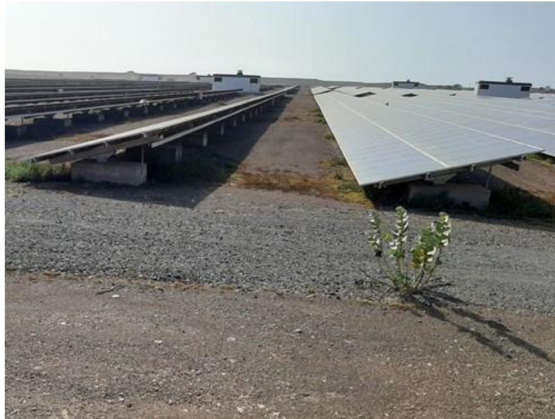
Photo 1 - Solar PV panels and support structure set in concrete blocks (Sal Island)
