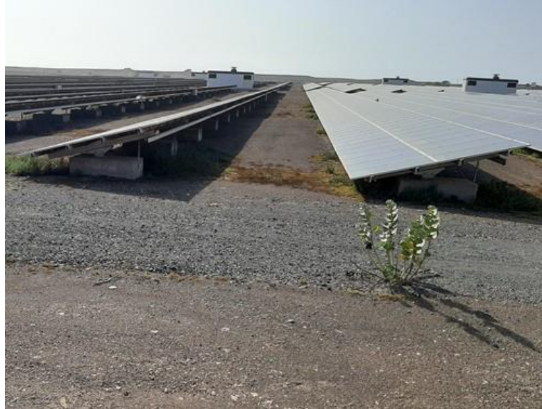
Photo 2 - Solar PV panels and support structure set in concrete blocks (Sal Island)
